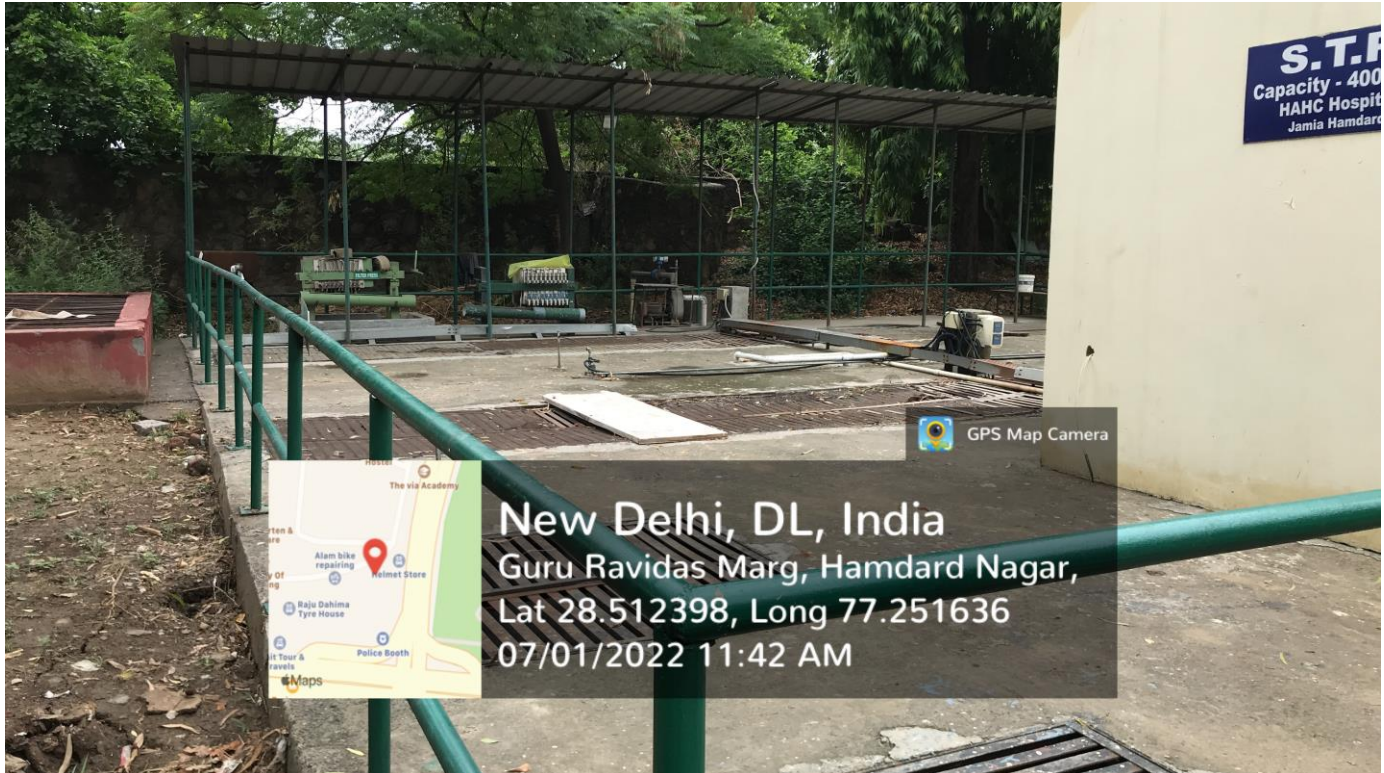
Sewage Treatment Plant
