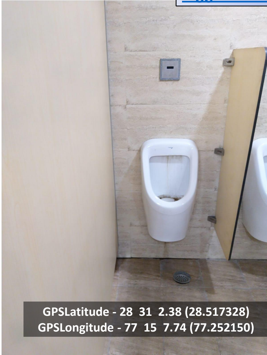
Sensor based energy conservation Washroom
