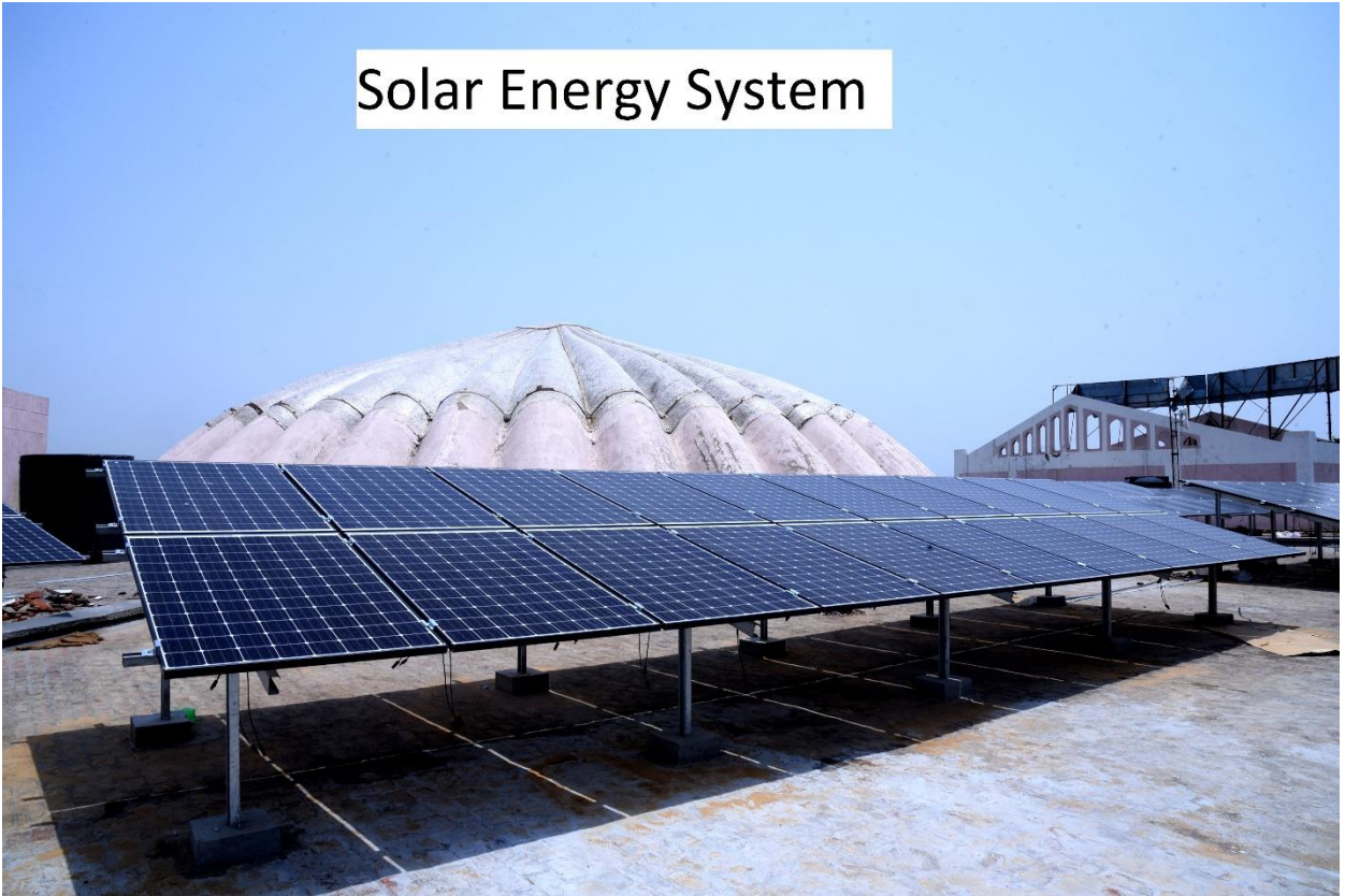
Solar Energy System
